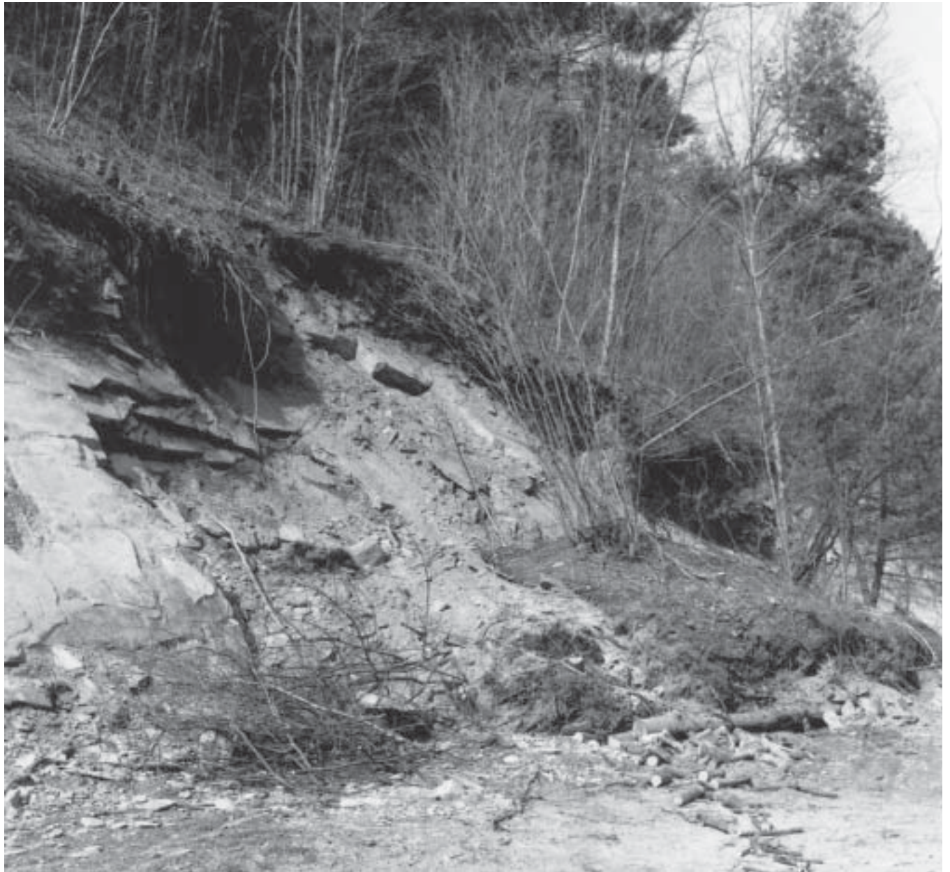
Figure 4.—Low-grade metasedimentary rock underlies soils such as Ditney, Unicoi, and Chestoa. This bedrock is unstable when lateral support is removed during construction of roads.
