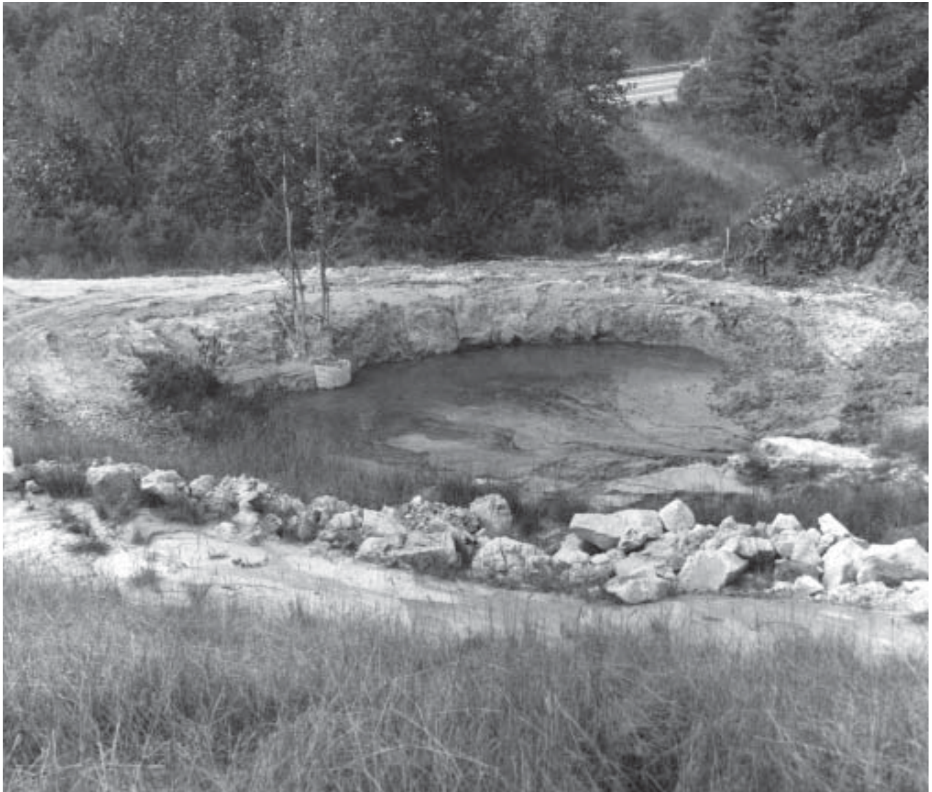
Figure 12.—Sediment basins should be installed before land disturbing activities begin. They keep eroding soil on site and help to maintain water quality.
